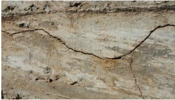
FIGURE 2: Cracks found on pile cap.
