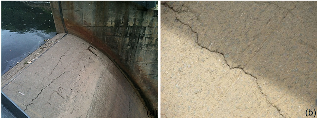
FIGURE 4: Cracks on the dam spillways – (a) and (b)
