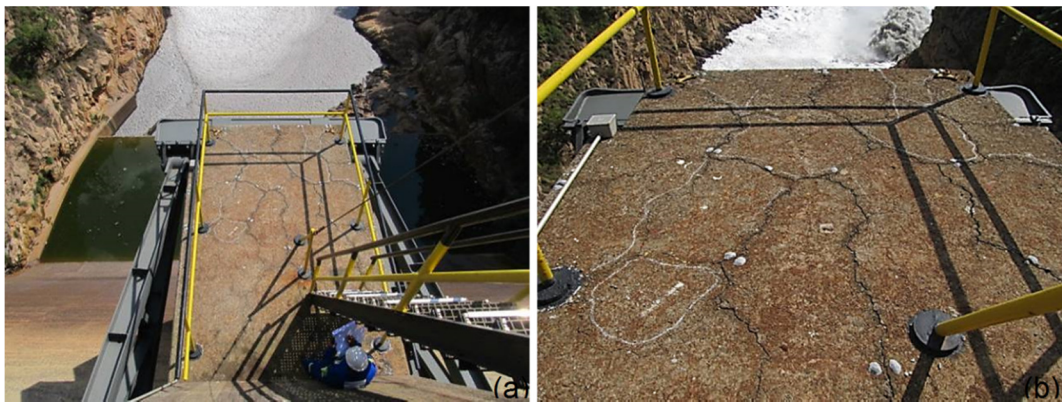
FIGURE 3: Map cracking chalk lined on the buttress top - (a) and (b).
