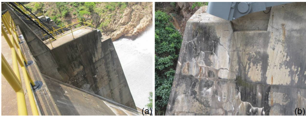
FIGURE 2: Map cracking and efflorescence of the buttress side (a) and trunnion beam area (b).
