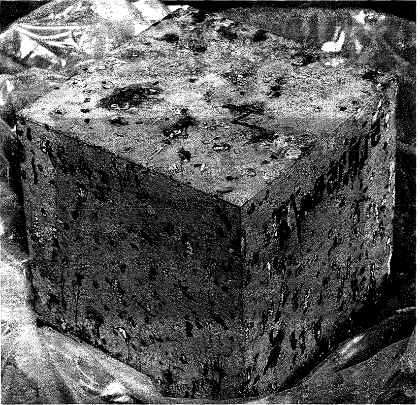
Deleterious alkali-aggregate reaction on a 30 cm sized cube which has immediately on demoulding been wrapped in foil
