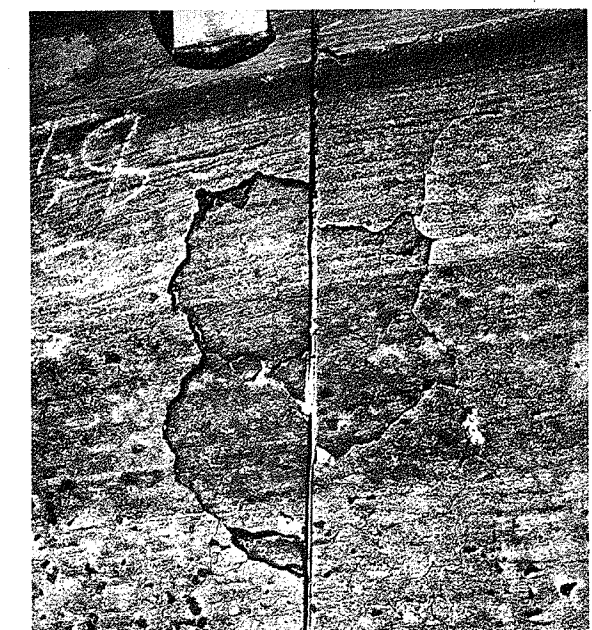
FIGURE 3: Typical appearance of a transverse joint after HVS testing.
