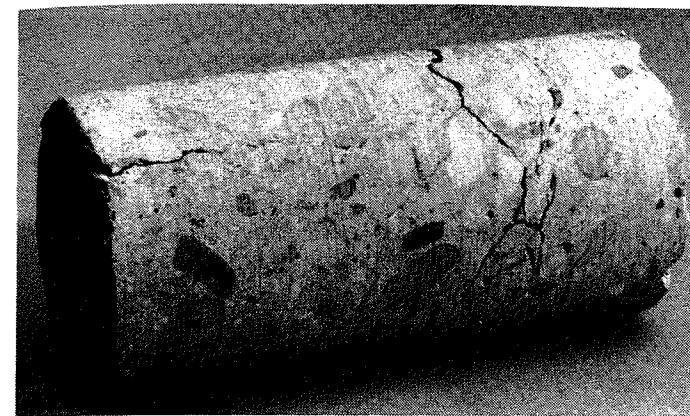
Fig. 4. Concrete core taken from the structure, showing deep cracks.
