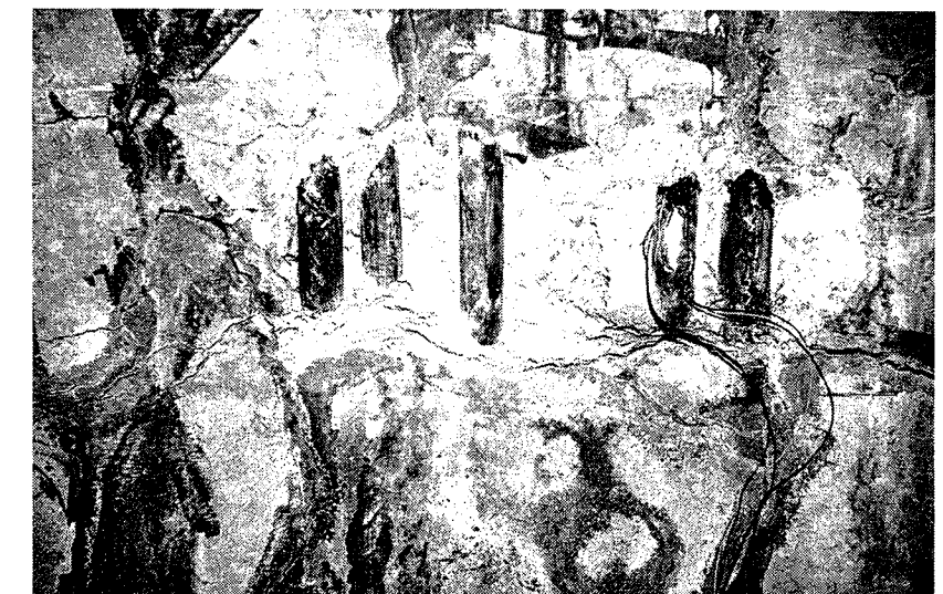
Figure 6. Main reinforcing bars in column exposed. Strain gauges mounted on second bar from right.
