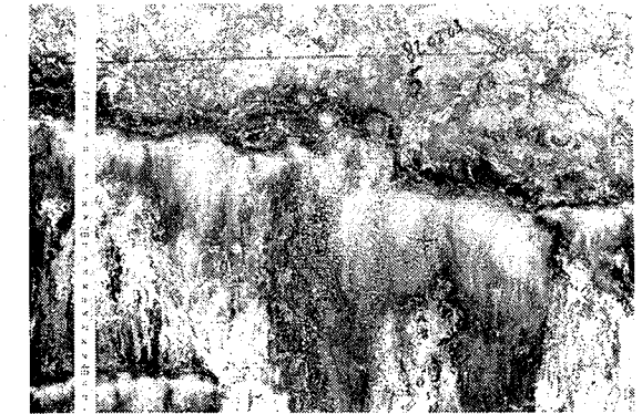
Note leakage around form tie
