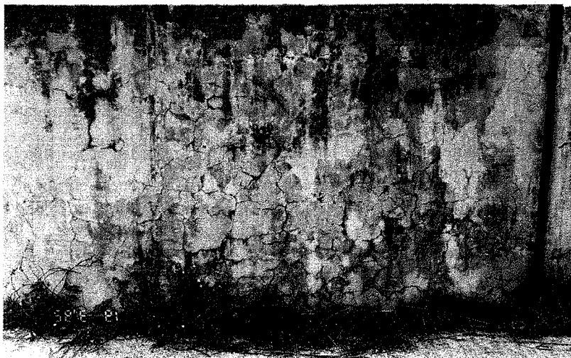
Figure 1 Map cracking on parapet wall
