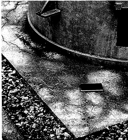
Figure 2. Cracking in a foundation block, age approximately 7 years. October 1976.
