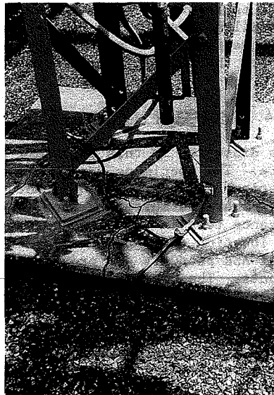
Figure 1. View of cracked foundation pier of electrical substation
