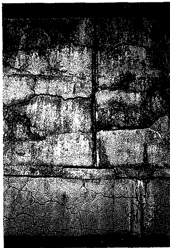
figure 5 Cracking in a retaining wall
