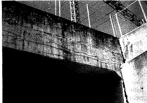
Figure 4 Cracking in a culvert box
