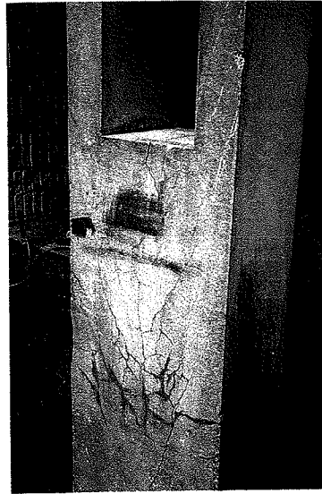
Fig. 6. : Detail of crack pattern.
