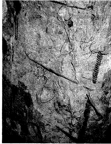
Fig. 3 Exposure of Steel Bar in Concrete
