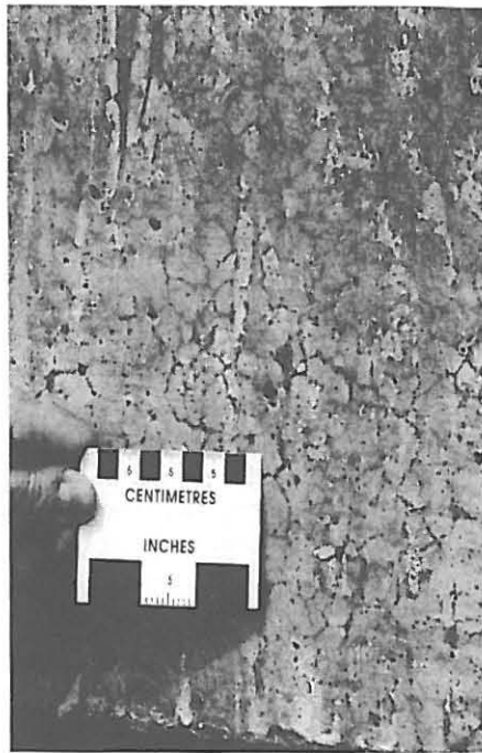
Fig. 5: Map cracking on Magpie River bridge
