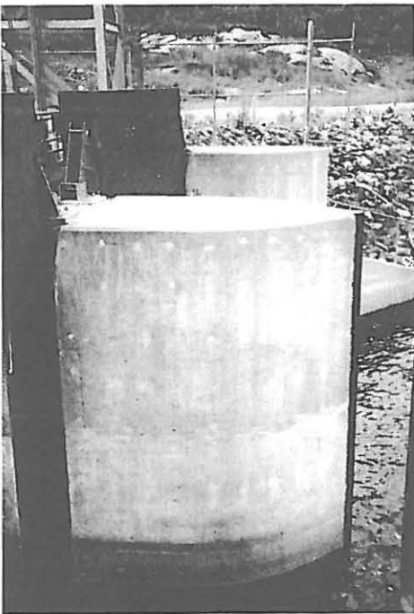
Fig. 4: Steephill Falls spillway (condition of spillway upstream pier, 10 years after construction)
