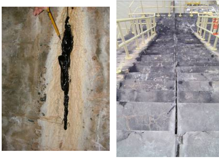
Figure 3: (a) Contraction joint with bitumen exudation (block B10-B11) and (b) Contraction joint between spillway piers at downstream with average 1 cm opening.
