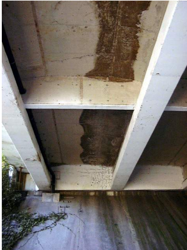
Figure 1: Dark patches on the lower deck surface.
