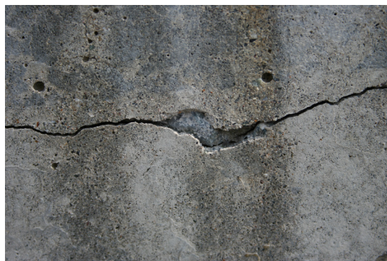
Photo. 2: View of scaling on concrete.
