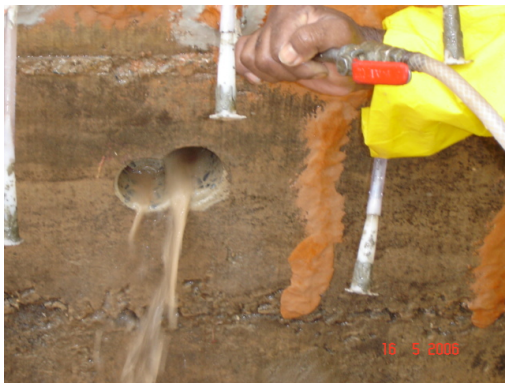
Figure 7: Washing of cracks using water injected under pressure and exit of dirt from the 2."-holes.
