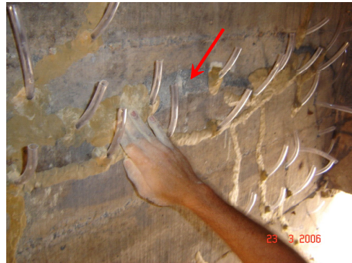
Figure 6: Superficial closure of the cracks and fixation of the purges using epoxy resin mixed with kaolin. The cracks closed with grout were also covered with epoxy (arrow).
