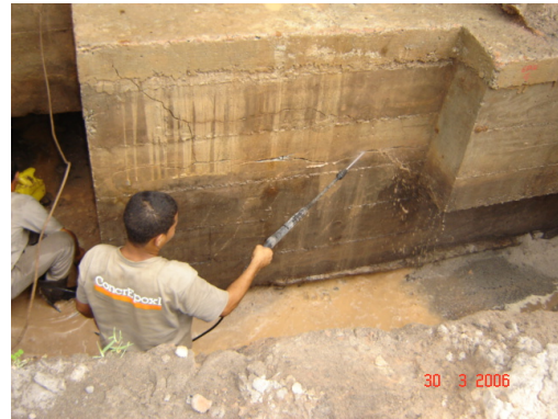
Figure 2: Cleaning of the block face using high-pressure washer, with a capacity of 400 kilopascal and flow of 360 liters/hour.
