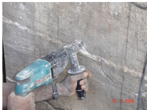
Figure 4: 1/2"-diameter and 4"-length holes using impact drill in cracks with smaller openings.
