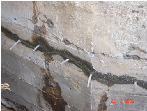
Figure 5: Non-fluid grout application in the cracks with opening larger than 10 mm and fixation of purges.
