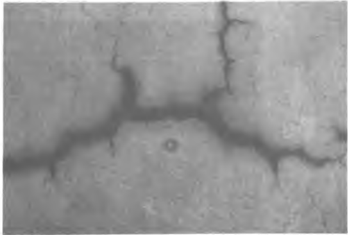
FIGURE 7 Cracking and staining of concrete due to extreme drying shrinkage
