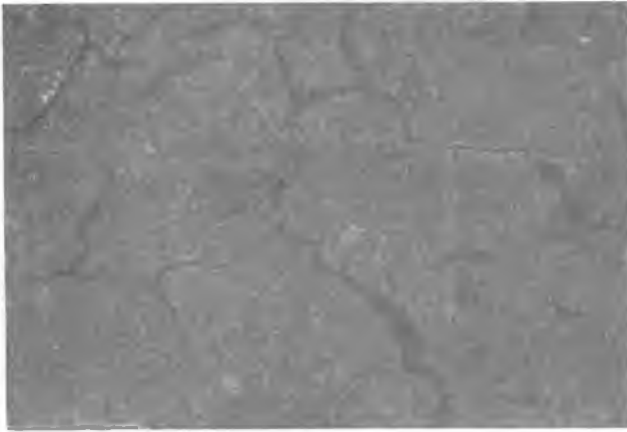
FIGURE 4 "Isle of Man" cracks on surface of concrete affected by alkali-silica reactivity (N America)
