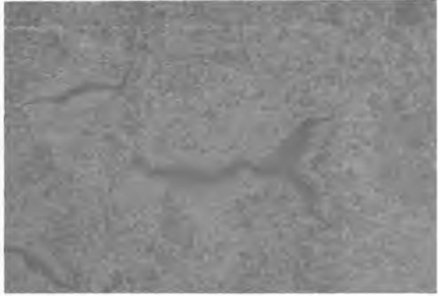
FIGURE 6 Cracking, gel exudation and staining of surface of concrete affected by alkali-silica reactivity
