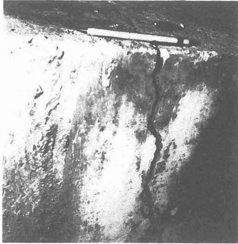
Figure 4: Typical crack in ARR-affected pier cap.
