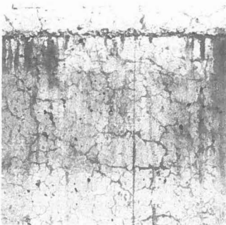
FIGURE 6 MAP-CRACKED 12 YEAR OLD CONCRETE
