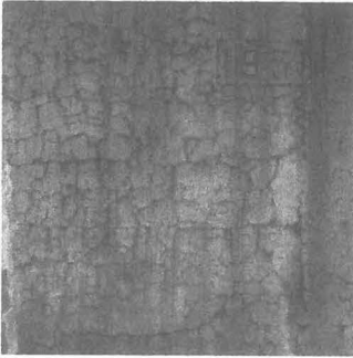
FIGURE 2 MAP-CRACKED 27 YEAR OLD CONCRETE
