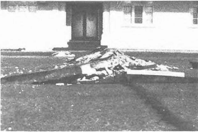
Fig.3 Strains built up over twenty years through alkali-aggregate expansion were abruptly released in and caused the damage illustrated.
