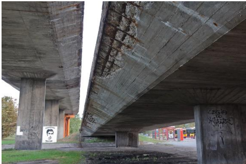
Fig. 1.1: Viaducts of Trasa Łazienkowska in Warsaw before demolition in 2012 with concrete spalling, corroded steel reinforcement, cracks and exudations, possibly due to ASR [4]
