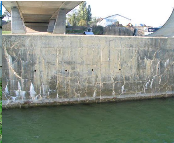
Figure 6.2: DEF damage from severe 1.5 to 5.5 mm/m variable expansions - (the white exsudations are calcite due to the dissolution of the lime of the cement and its carbonation with air).
