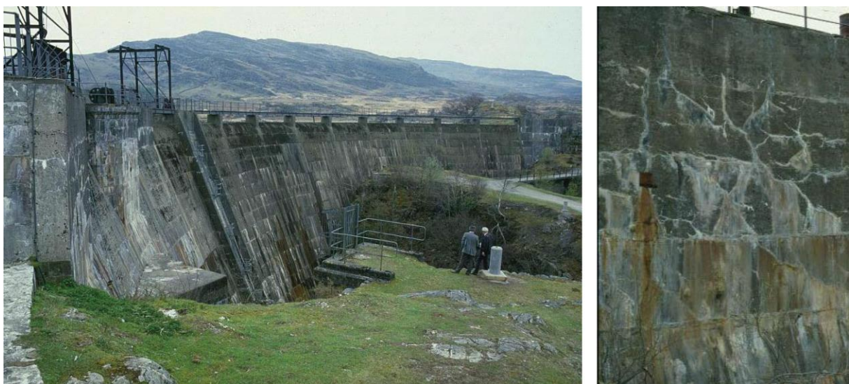
Figure 2.2: Maentwrog Dam, North Wales (left), showing cracking caused by ASR, but also suffering long-term water leaching and localised freeze-thaw damage (right).
